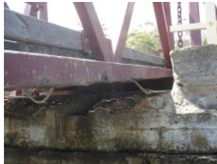
Corroded sections of bottom steel member of gangway
