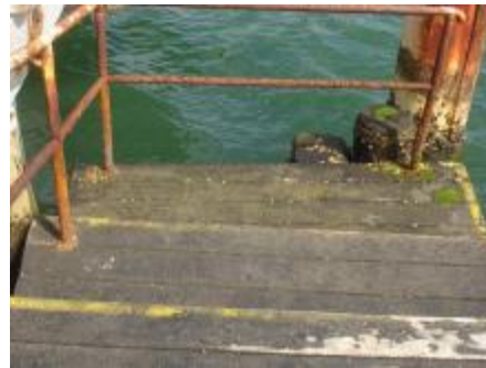
Stairs with patchy antiskid treatment and some marine growth.
