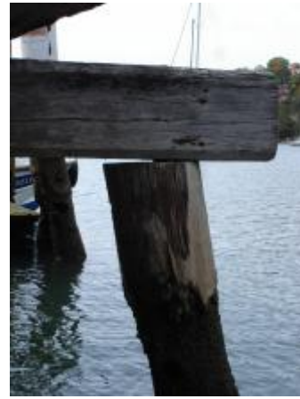
Headstock bearing unevenly on pile
