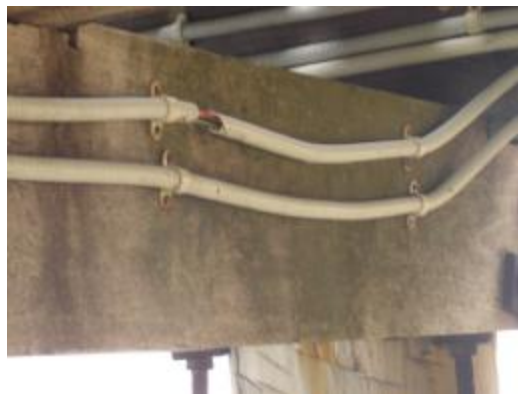
Exposed wires are unsafe
