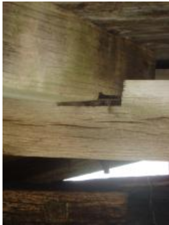
Girder bearing unevenly on headstock
