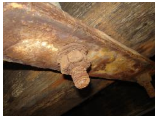
Delaminating bolt connection
