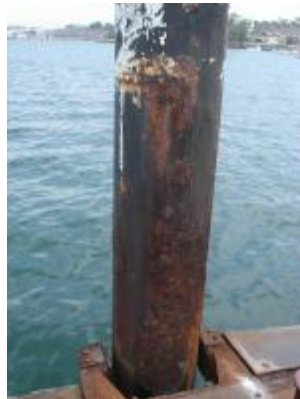
Steel pile with some corrosion
