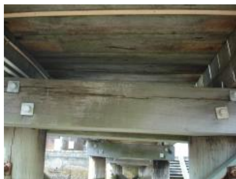
Horizontal mud leads evident of termite presence
