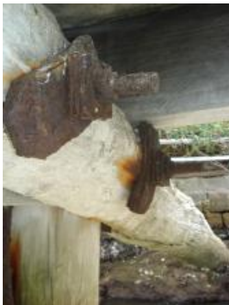
Bolts beginning to delaminate
