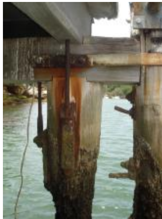
Loss of cross-section evident from this corroded pile/headstock connection
